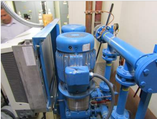
View of the two booster pumps
