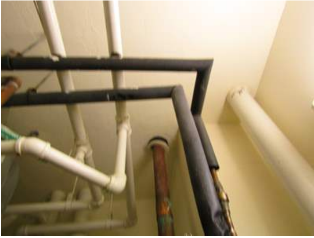
View of water supply lines and drain lines
