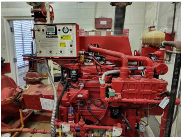
View of the fire pump
