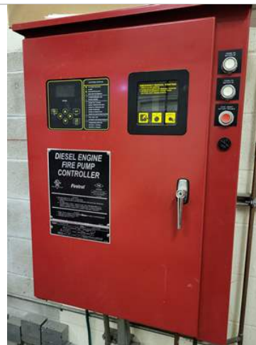
View of the fire pump controller
