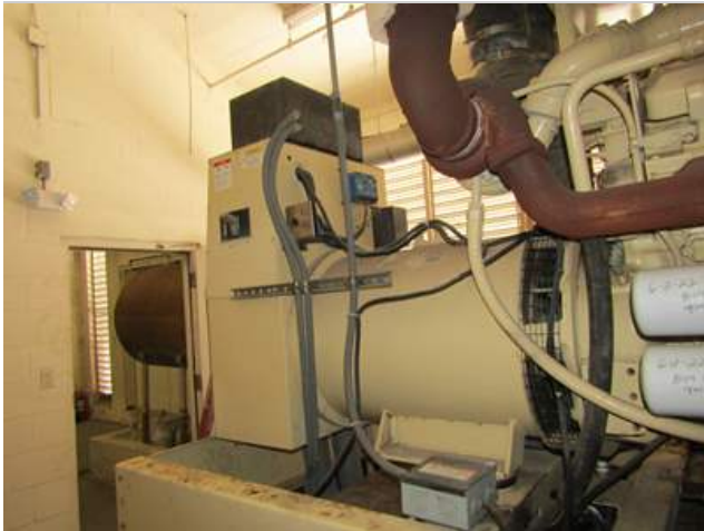
View of the emergency generator
