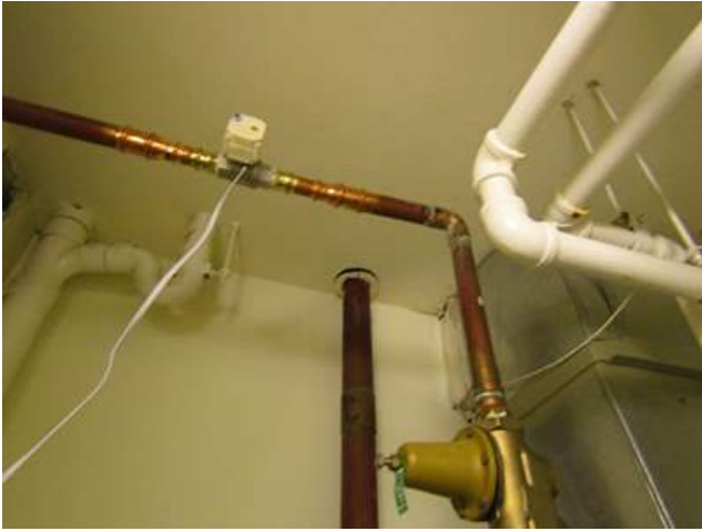
View of water supply lines and drain lines
