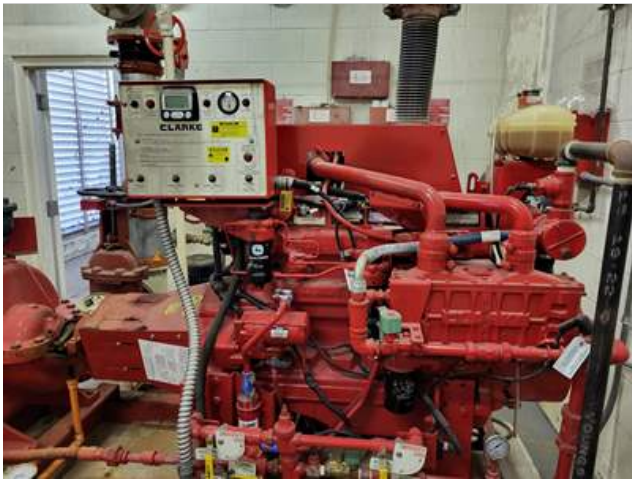
View of the fire pump
