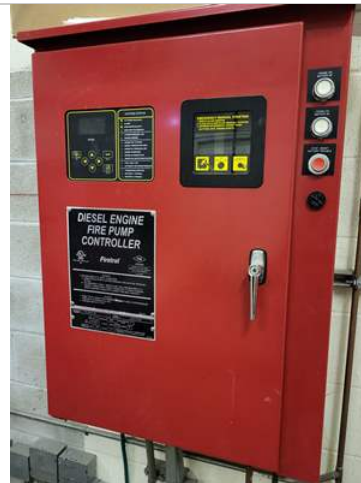
View of the fire pump controller
