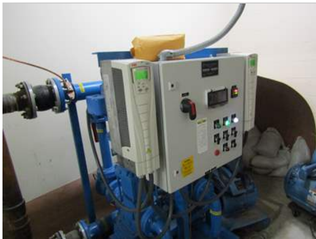
Domestic water pump controls
